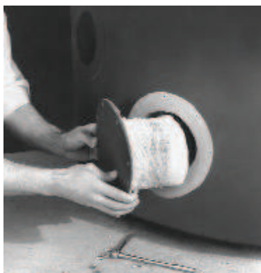
FIGURE 8 - REMOVING CLEAN OUT PLUGS
